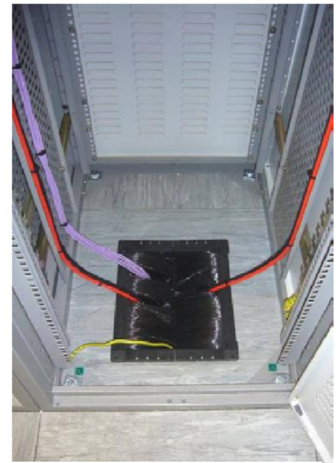
Brush strip grommet now supplied and fitted with all rack installs
